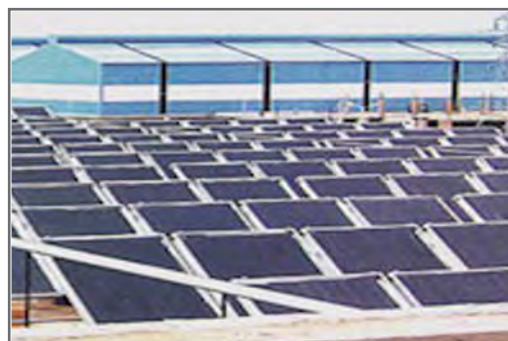
Fig 3.15: Solar Panels to trap solar energy
